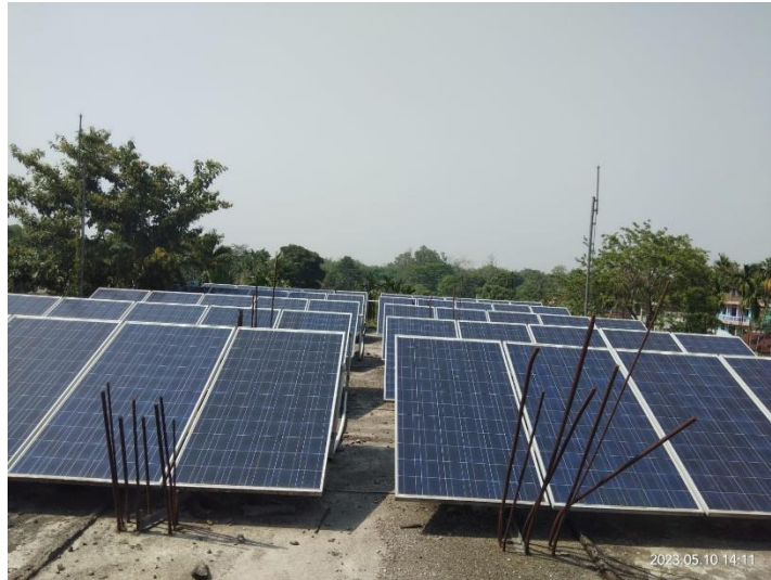
Figure 11: 10 kWp Solar Power Plant installed in the campus
