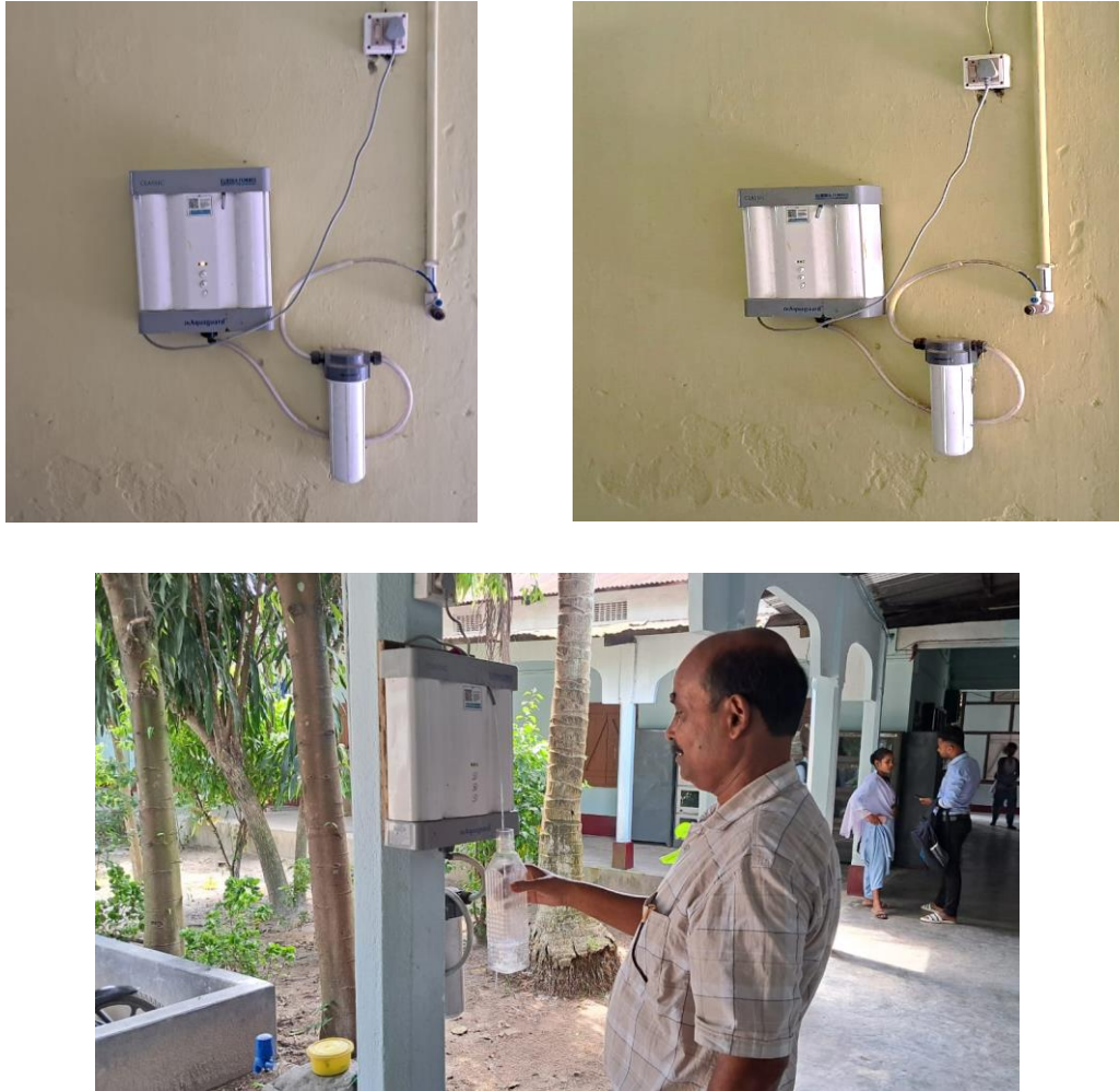
Figure 3: Water Purifier installed in the campus
